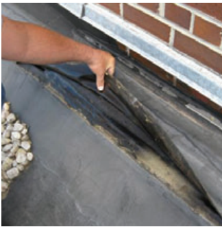
❑ Failed single-ply flashing
