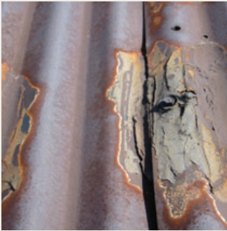
□ Rusted metal roof with fastener deterioration
